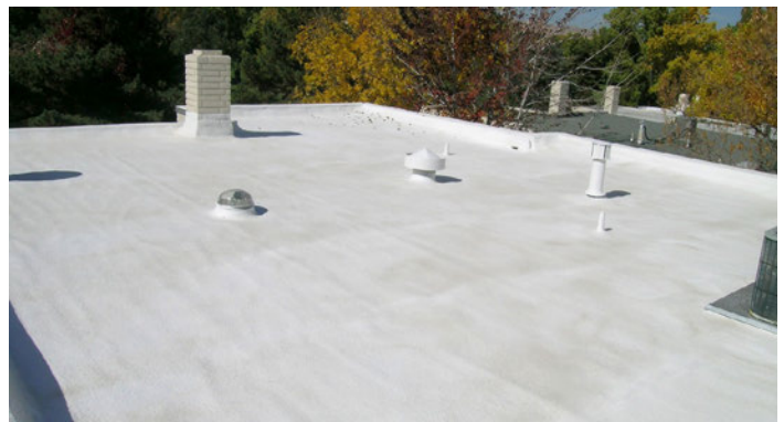
Cool roofing material
