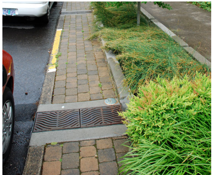
Bioretention planters for stormwater management, Portland OR
