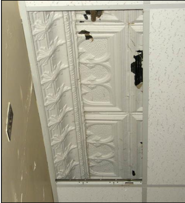
Image 15: Interior ceiling of the 1872 one-room schoolhouse, showing moulded tin ceiling tiles and crown moulding, later obscured under a drop-ceiling. (Image Date: February 24, 2011)
