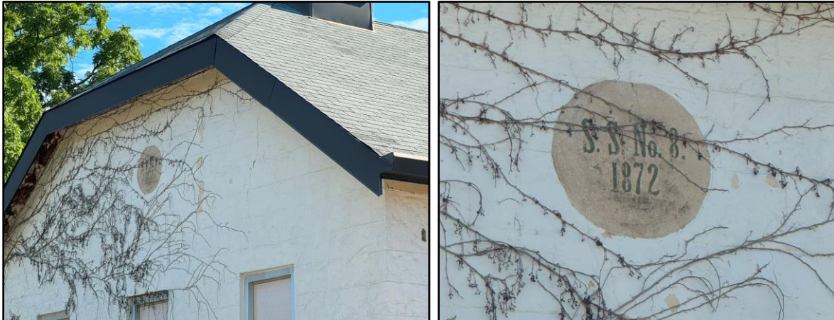
Image 3a & 3b: Detail, jerkinhead roof profile of the primary façade (south elevation) of the 1872 one-room schoolhouse, and a detail of the date marker reading “S.S. No. 8. 1872”.
