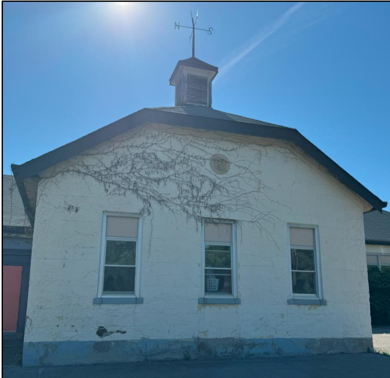
Image 1: Primary Façade (south elevation) of the 1872 one-room schoolhouse. (Image taken on: June 28, 2024)
