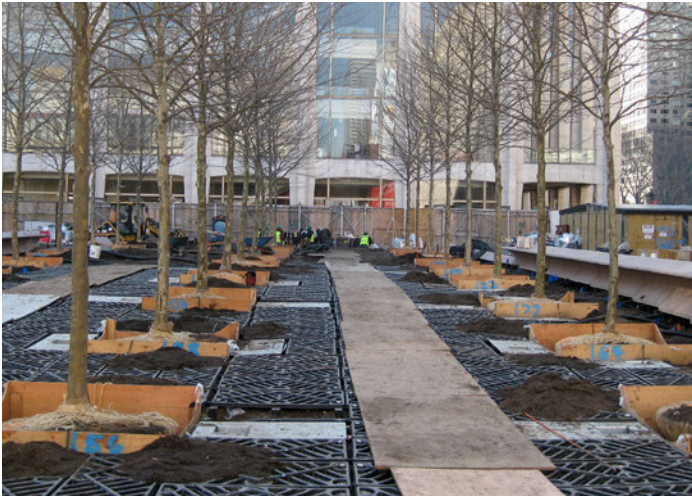
Soil cell installation at Lincoln Center New York (Source: DeepRoot on Flickr.com)
