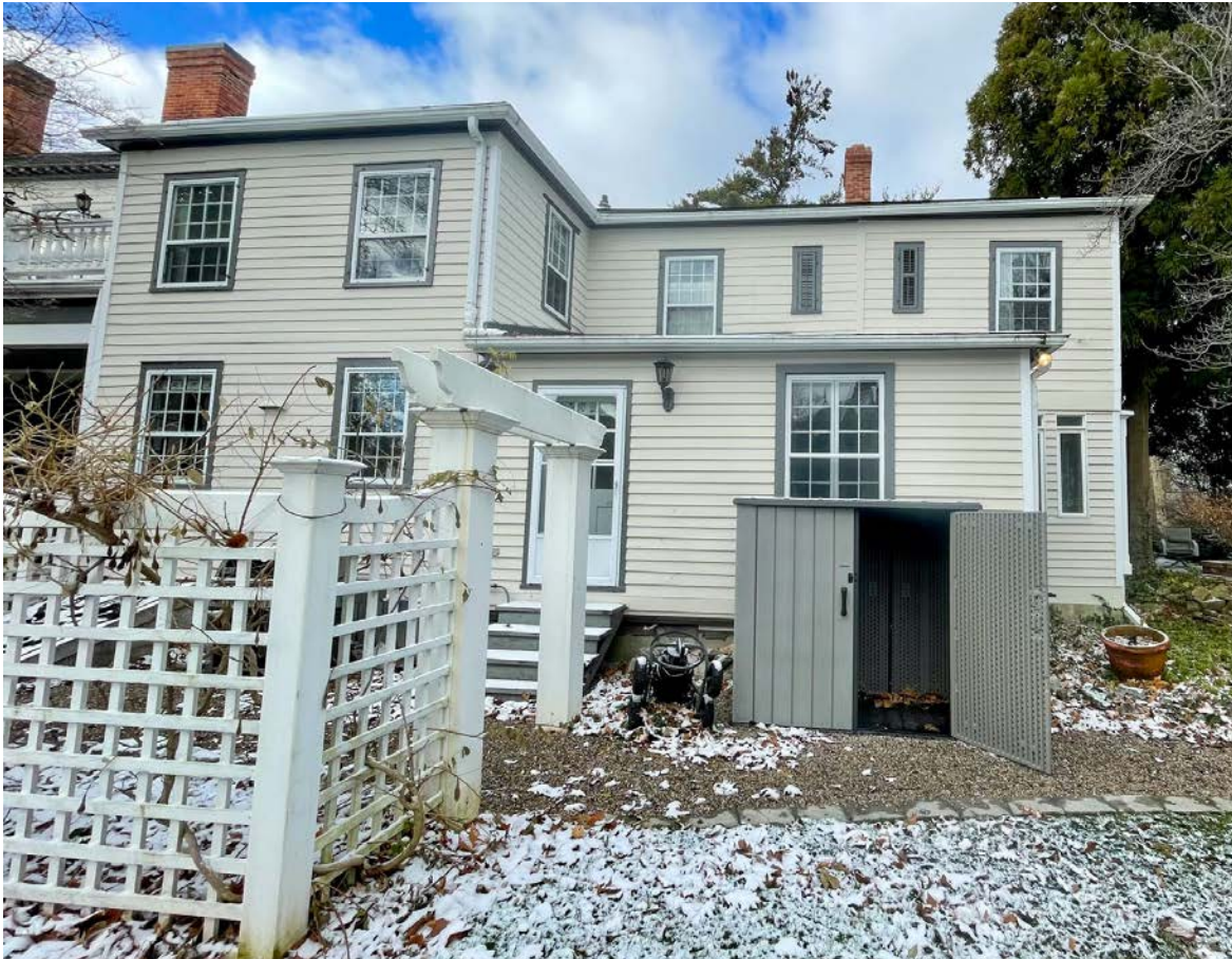
REAR ADDITION – the rear addition with a secondary door that enters into coatroom
