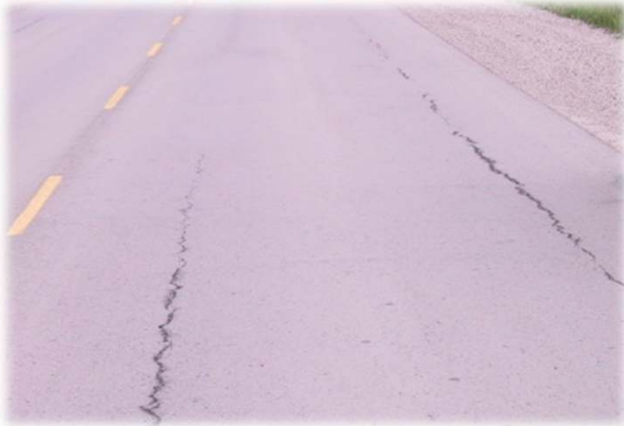
Figure 3: Wheelpath Fatigue Cracking
