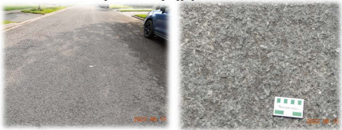
Figure 3.3: Ravelling / Aggregate Loss
