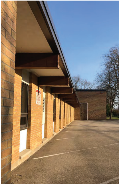
17. View of the south elevation of the 1956 addition and part of the north elevation of the 1976 addition (Source: ERA Architects).
