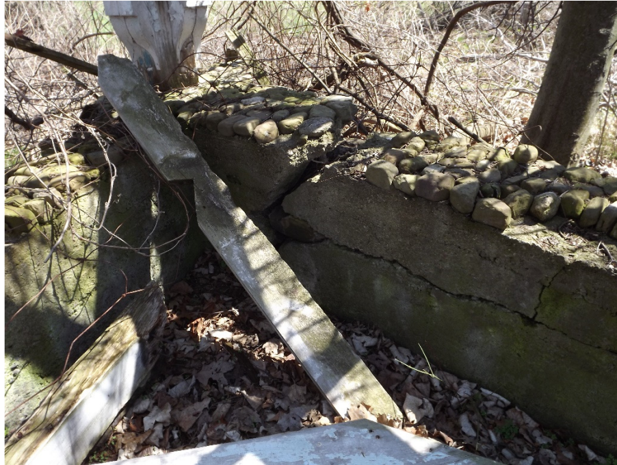
Broken and displaced wall and rafters, northeast corner
