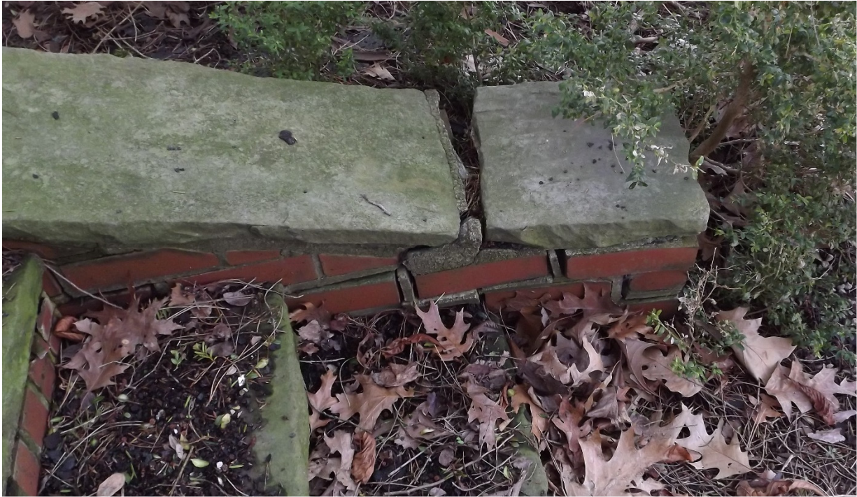
Failed parapet wall on rear stairs
