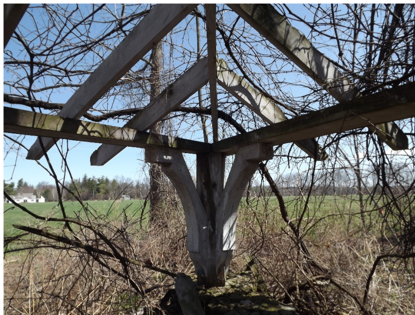
Intact but deteriorated framing, northeast corner
