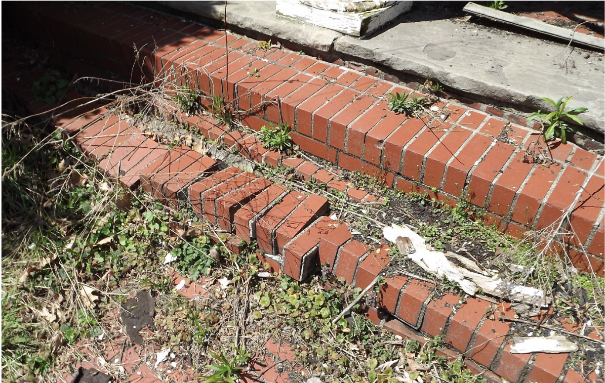
Collapsed brick steps
