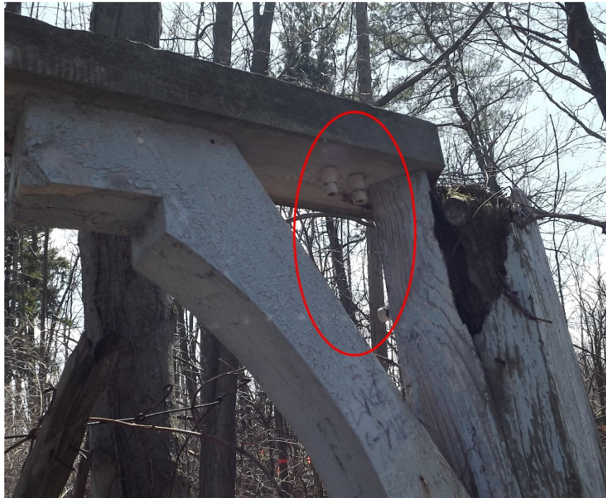
Porcelain electrical insulators beside south entrance
