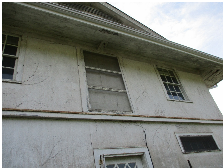
West end, trims need minor work and paint, hay loft door with hook above
