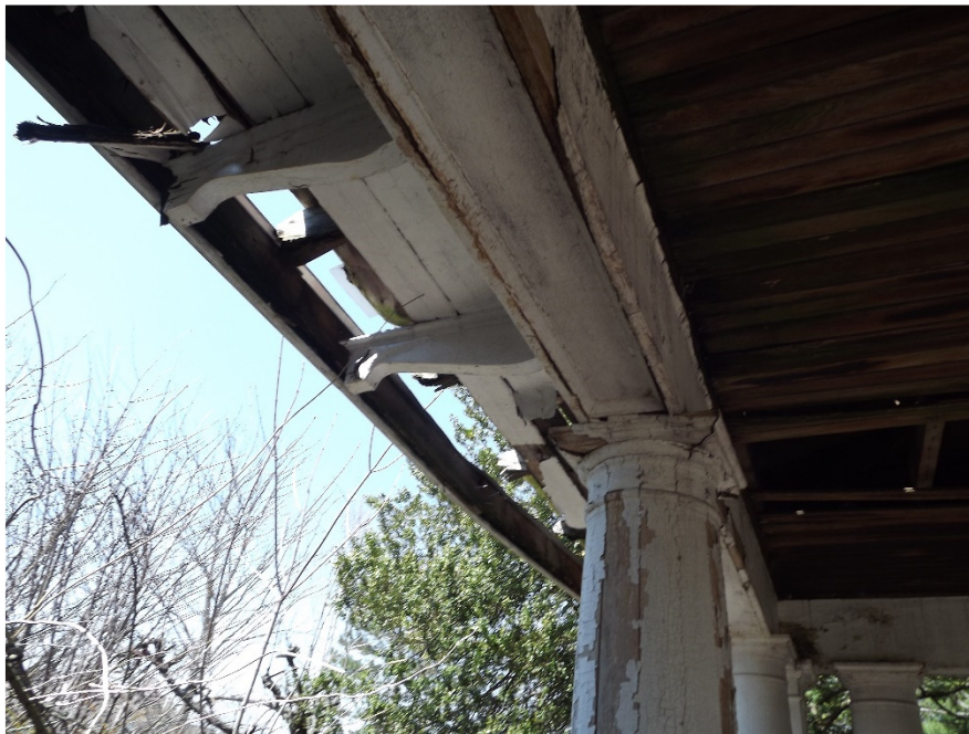
Section of eave requiring replacement
