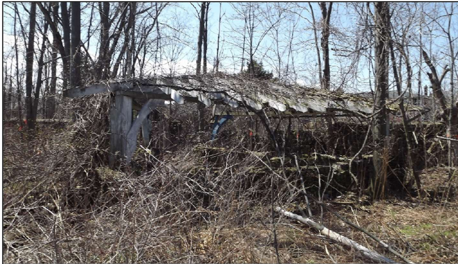
Figure 27 - Whistle Stop gazebo with roof partially intact, April 2022, in Shoalts Building Condition Assessment – Whistle Stop, p. 3.
