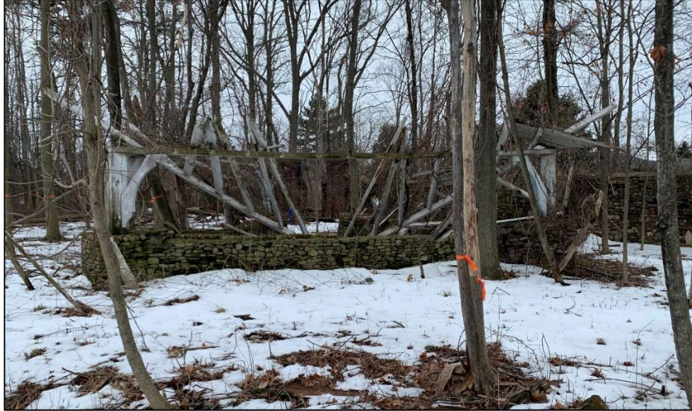
Figure 1 - Whistle Stop Gazebo with collapsed roof, March 2023.
