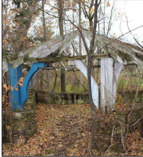
Figure 26 - Whistle Stop in 2018 with roof structure mostly intact. Source: LHC CHER 2021, 200 John Street East, p. 93.
