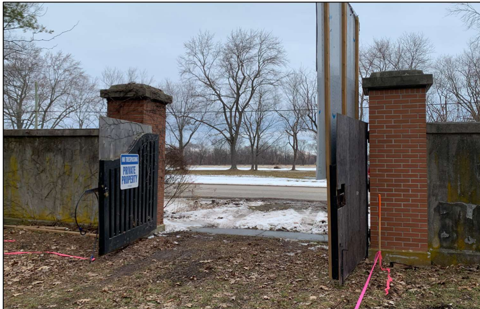
Figure 14 - Brick entrance pillars and boundary wall at entrance, 200 John Street East, March 2023.
