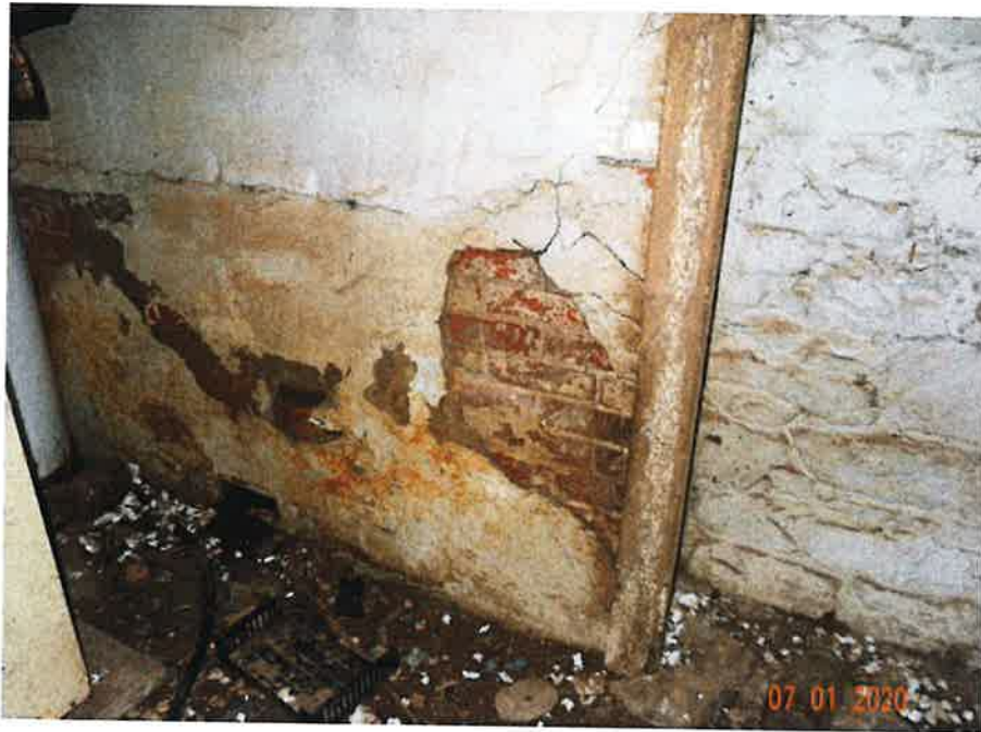
Figure 21: Concealed Basement Cooking Oven
