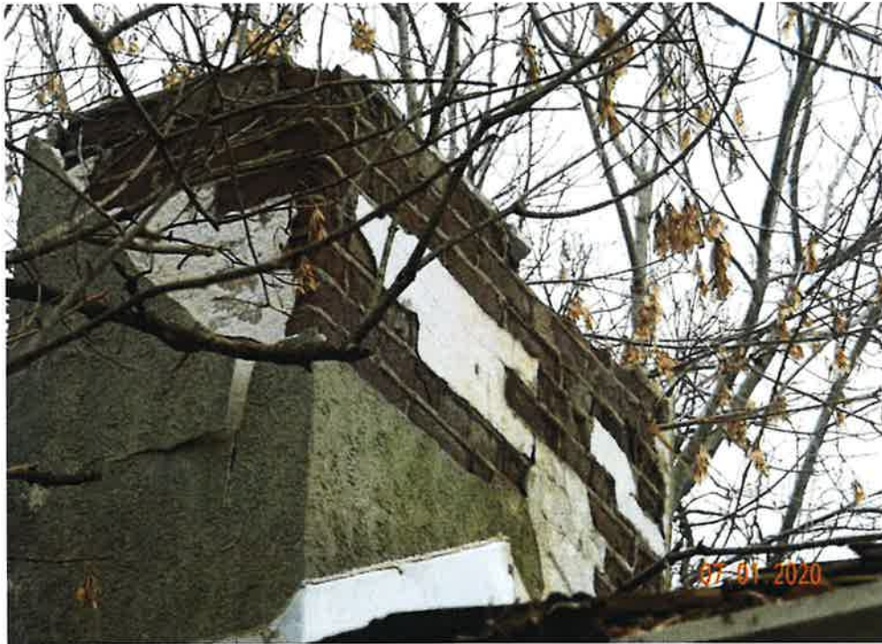
Figure 4: Chimney with Failing Stucco, Brick Exposed
