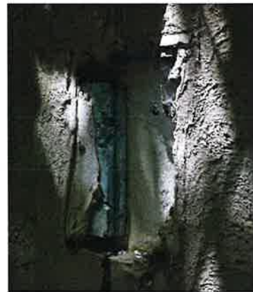
Opening in stucco finish, revealing foam insulation and earlier stucco finish. (ERA)
