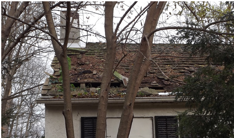
Front roof with holes
