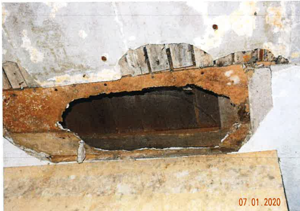
Figure 12: Ceiling with Exposed Lath and Floor Boards
