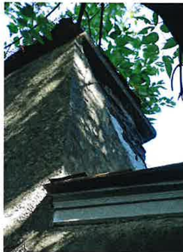
Deterioration of chimney brick and stucco (ERA)
