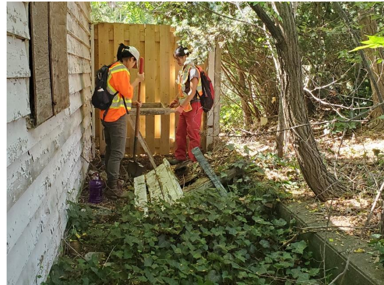
Image 14: View of test pit survey conducted to within one-metre of the extant garage.
