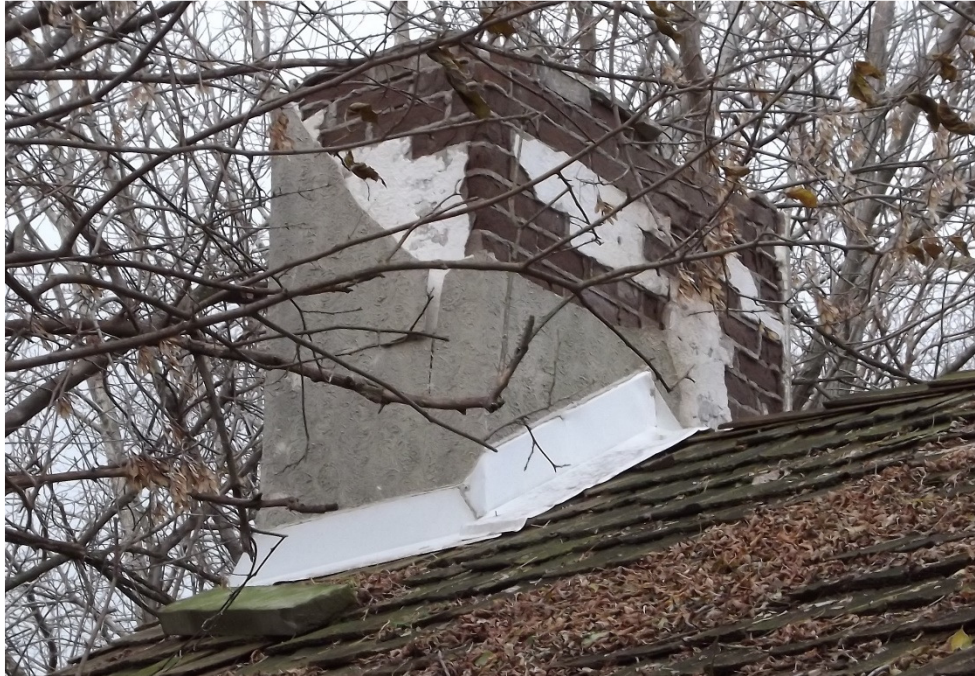
Chimney with cap fallen off, failed stucco, and failed brick
