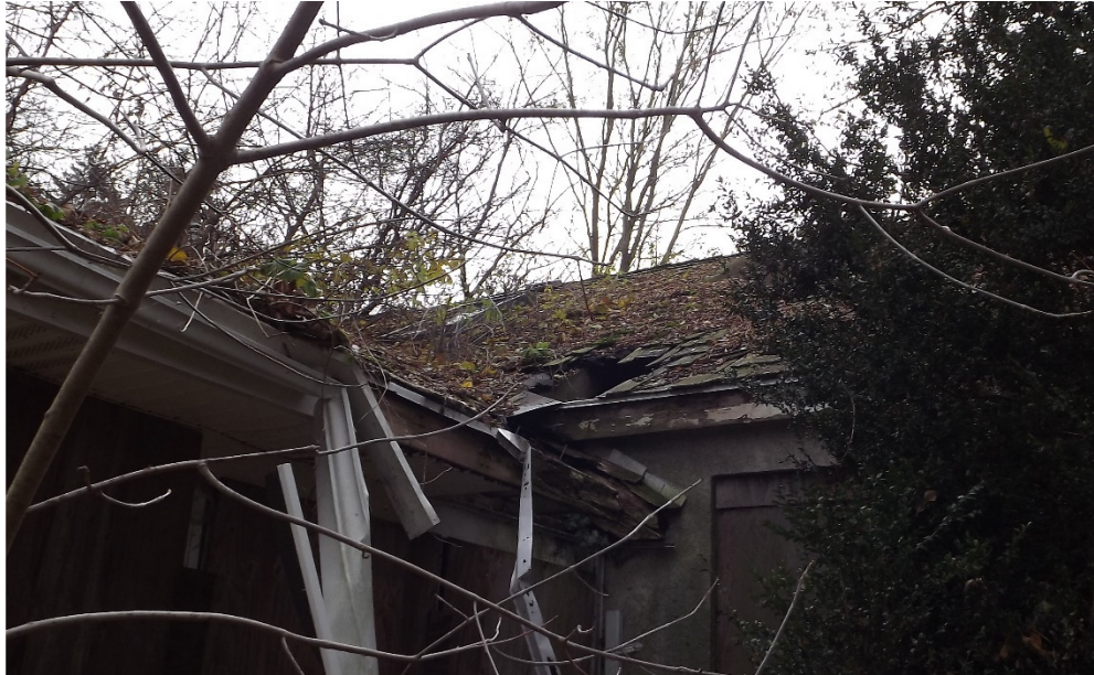
Rear roof with holes
