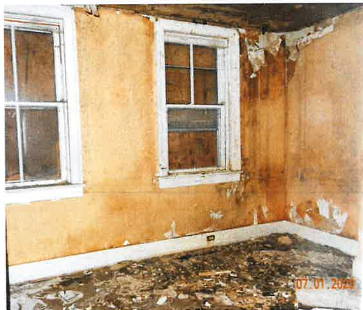
Figure 8: Boarded Windows, Peeling Paint and Mould
