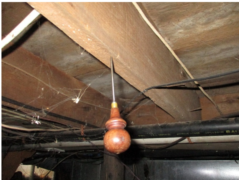
Deteriorated floor joist, awl inserted >2"
