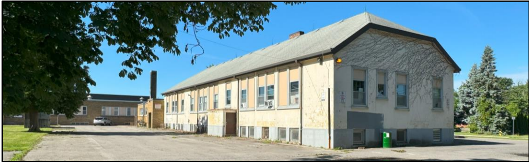
Image 8: West and north elevation of the first phases of expansion of Virgil Public School. The 20 th century addition has basement windows, and models the style of its opening and roof profile, albeit on a larger scale, from the 1872 design. In the distance, a subsequent addition clad in buff brick is visible. The land surrounding the building is paved. (Image taken on: June 28, 2024)
